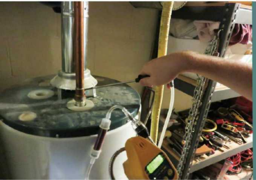
Flue gas CO testing with attached NO x filter
